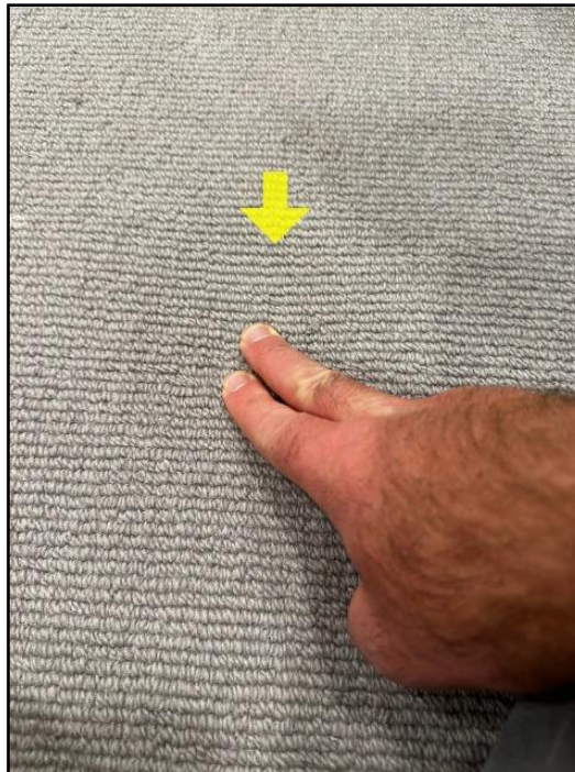
Post inspection photo - Drain under carpet
