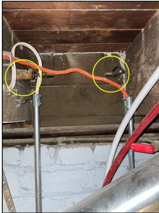
Remnants of knob-and-tube wiring
