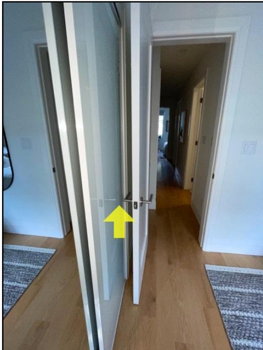
Example : At Second Floor Front Bedroom
