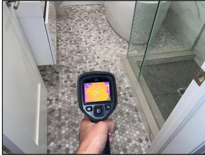
Radiant floor heating (electric)
